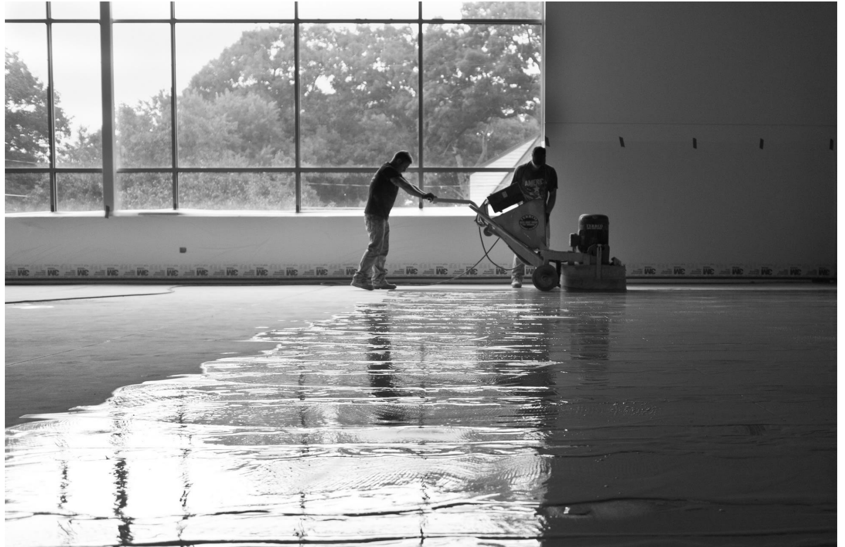
Finishing the Floors; Polishing the concrete flooring inside the Jesse Franklin Taylor Education Center construction site.
