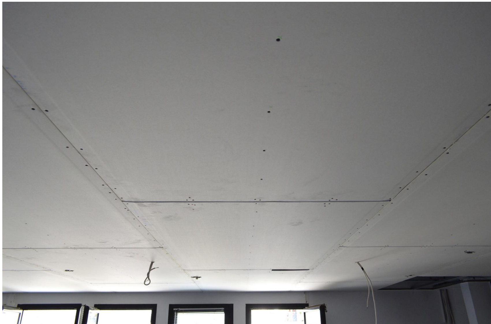
"Installing plasterboard ceiling" by 1st floor renovation of Veria Central Public Library. [c] All rights reserved via Flickr
