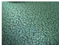
Cracking due to chemicals
