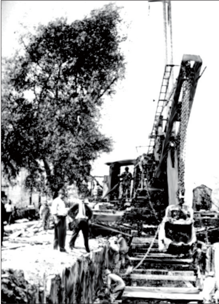
Photo II.8. Sewer construction, 1910. Source: Leonard Metcalf and Harrison P. Eddy, American Sewerage Practice: Volume II Construction of Sewers (New York: McGraw-Hill, 1915).
