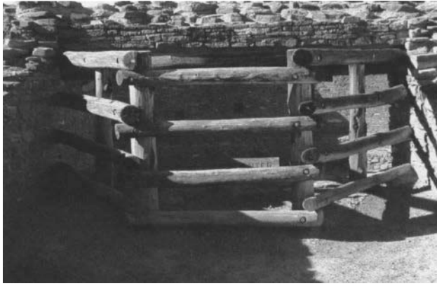
Gate blocking the entrance to Casa Rinconada. Today access to the interior of the kiva is blocked by these barriers. From the rim above, visitors can see the kiva, including the floor features, which were obscured in the past. The uncovering of all the architectural features can contribute to the understanding of the visitor. However, the ban on access required for the protection of the ruins prevents visitors from experiencing the space of the kiva. Photo: Marta de la Torre
