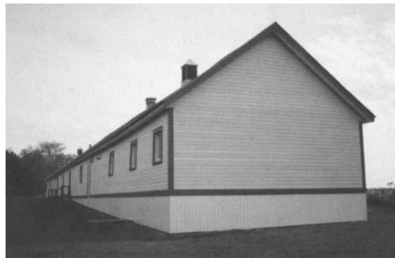
The west end and rear of the Lazaretto, showing some of the windows and doors in the back wall of the building, as well as the bead-board skirt that covers the replaced piers that support the building.
