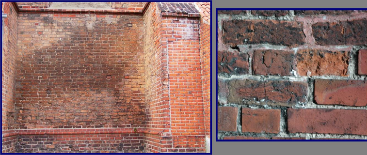
Fig. 4 Brick wall – deteriorated bricks were replaced by the new ones, Chelmno St. Mary Church (J. W. Łukaszewicz)
